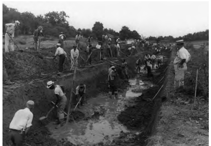
In 1940, the federal Works Progress Administration paid day laborers to dig the trench in which the Beals Branch sewer would be constructed.
