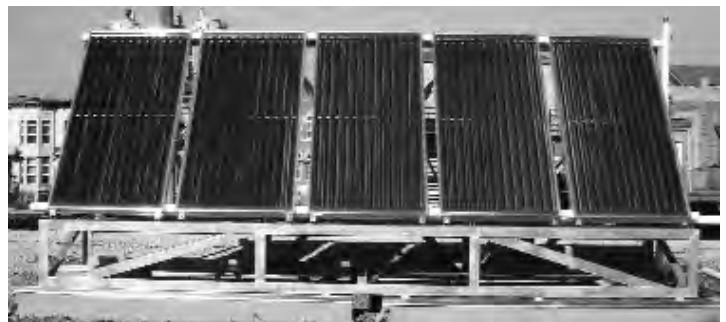
Solar hot water collectors on the roof of a fire station in Chicago. Photo: Andy McDonald
