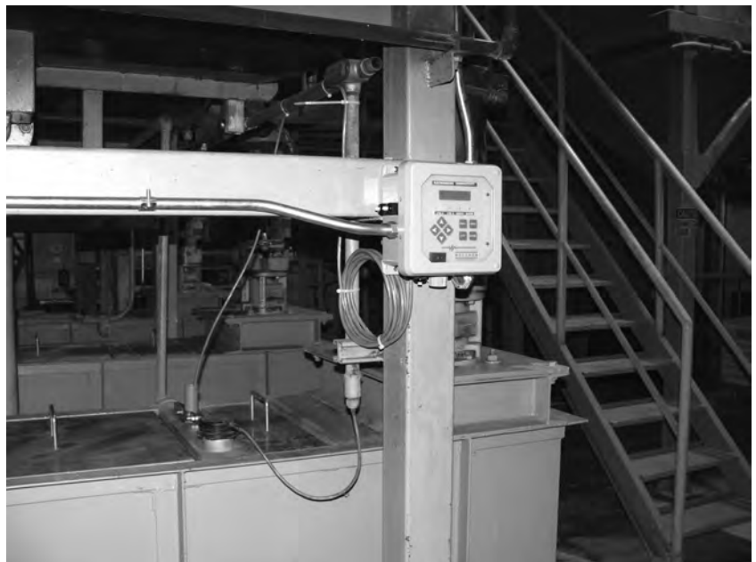
A non-contact, toroidal controller installed on a plating line resulted in significant savings in water, labor, wastewater treatment chemicals and sludge disposal.
