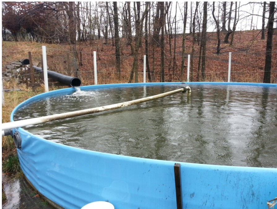
Figure 17: Primary tank for collecting stormwater runoff
