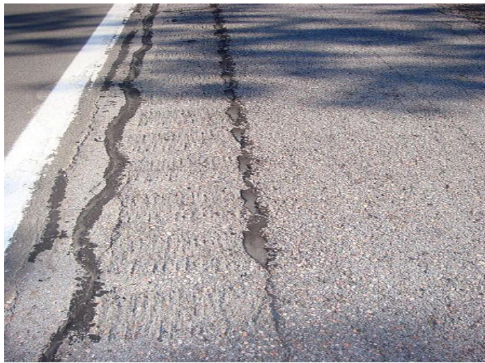
Figure 3-3 A typical example of out of section
