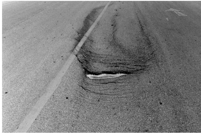
Figure 3-2 A typical example of other cracking
