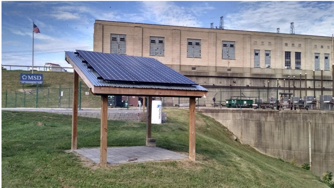
Figure 3.2 Panels for Powering Water Pump
