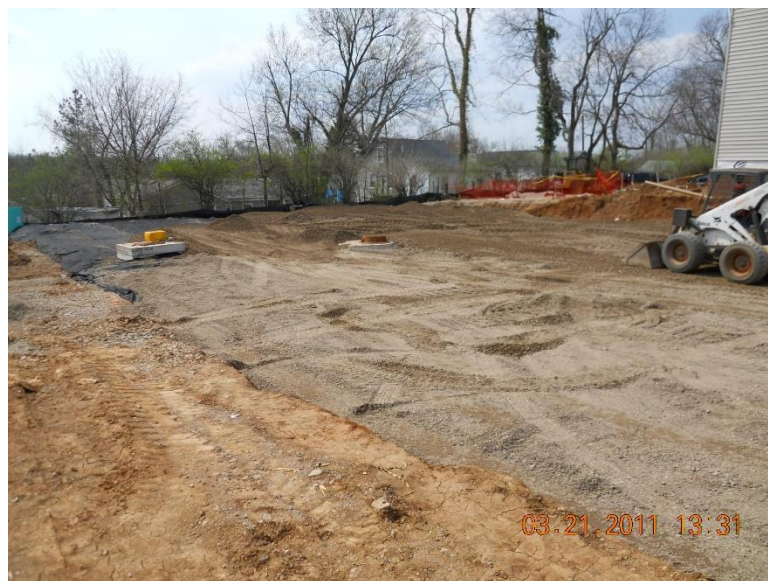
Figure 13. The basin is covered with Dense Graded Aggregate (DGA) and ready for the asphalt layer to be placed.
