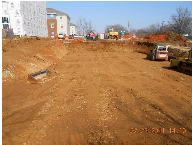
Figure 9. The basin has been excavated to the proper depth (954.5 ft. in UGF-1 and 955 ft. in UGF-2).
