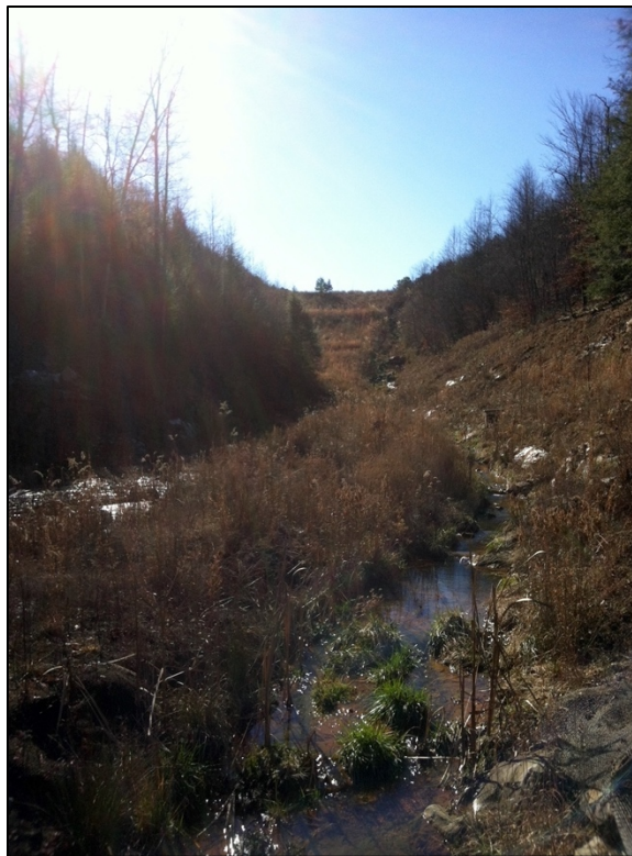
Figure 3. The Guy Cove valley fill viewed from downstream. The original headwater stream was at the bottom of the ‘V’ shaped fill. The created stream was constructed on top of the valley fill and establishes a ‘natural’ connection between the unmined upper watershed and the lower watershed downgradient of the valley fill.
