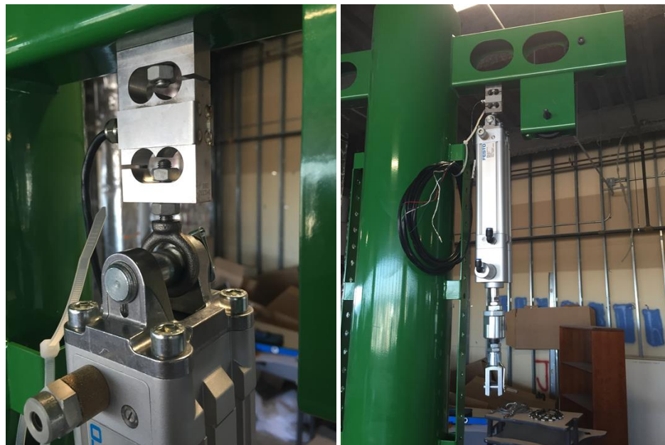
Figure 4.55: Installed Load Cell (Left) and Pneumatic Small cylinder (Right)
