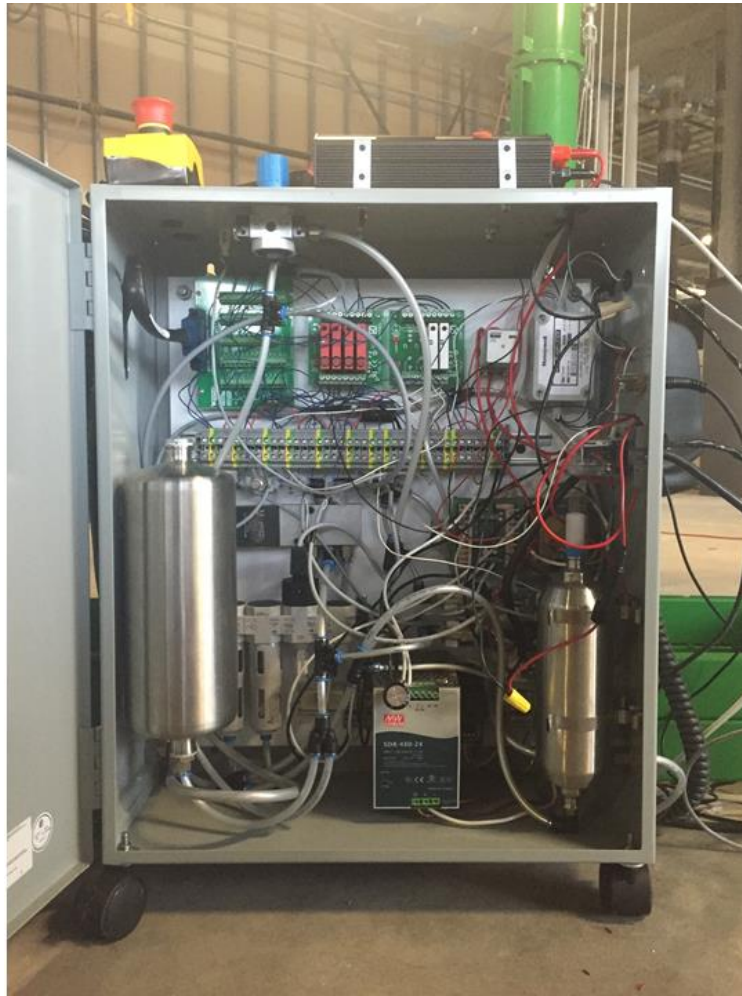
Figure 4.52: Completed BWST Pneumatic and Electrical Control System
