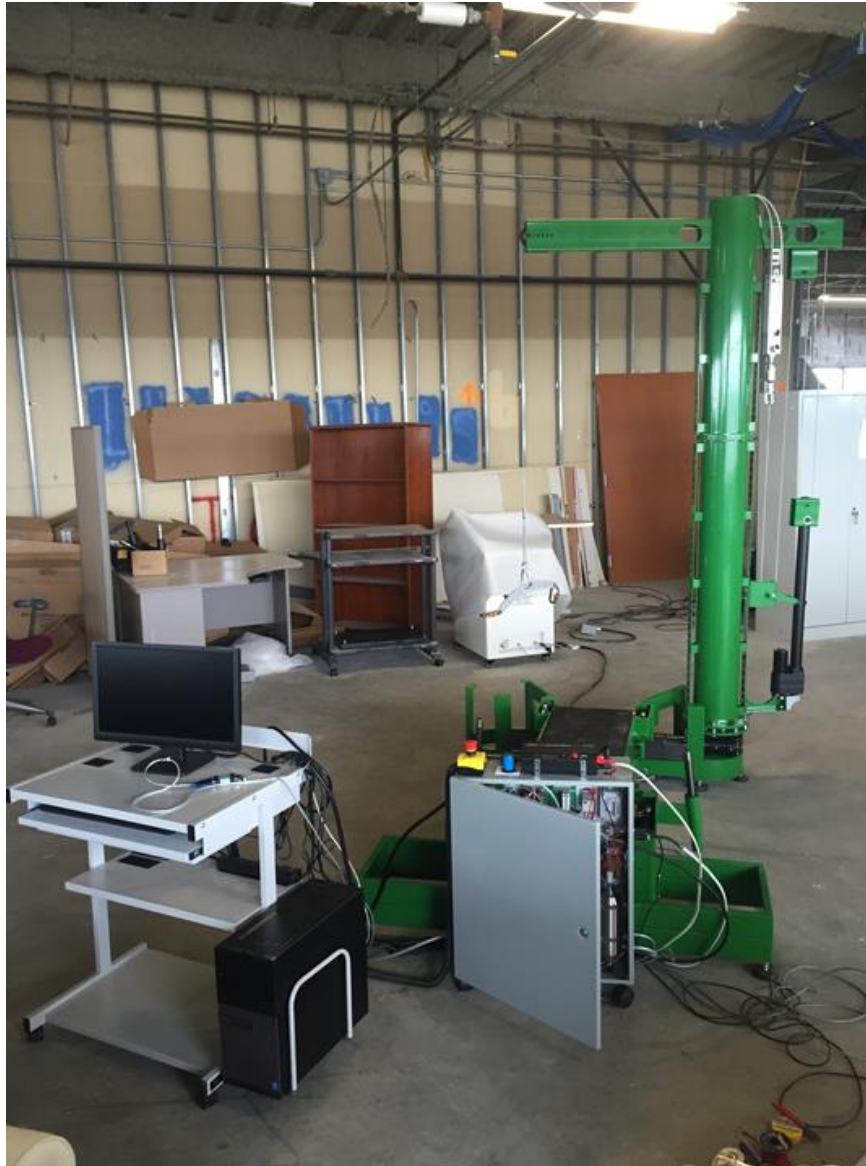
Figure 4.49: Installed Complete BWS, Control System, and Computer
