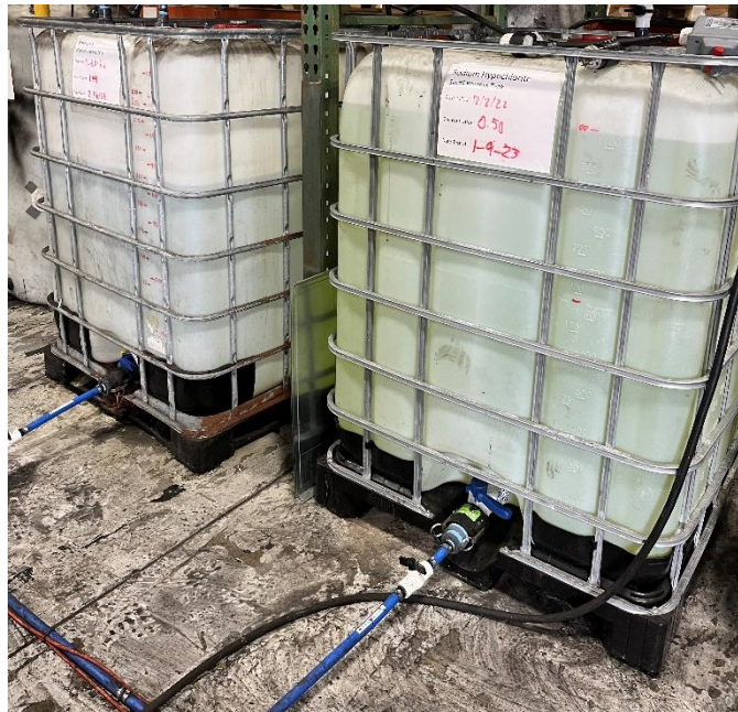
Figure 21 - Bleach and Ammonia Storage at Arduro Pilot Plant
